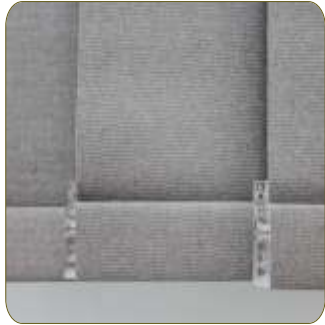
Front View of Panel Bottom
